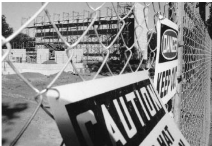
The $2 million renovation project at Hale School Began in July and will be completed next fall,. The north wall of the new gym begins to take shape in the background.
