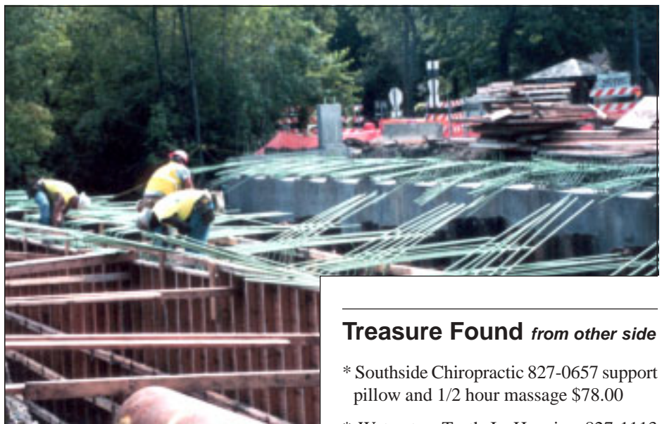
Iron workers installing steel rebar on the north side of Minnehaha Creek.
